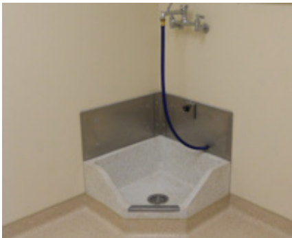
Typical Mop Sink
