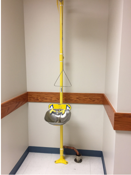
Typical Emergency Eyewash and Shower Equipment Station
