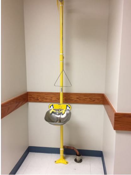
Typical Emergency Eyewash and Shower Equipment Station
