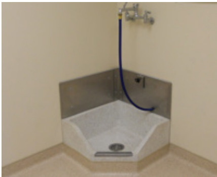
Typical Mop Sink
